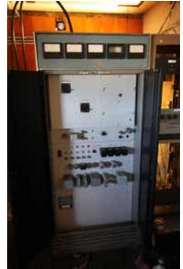
The CCA 1000-D before its removal from the old WABY studio/transmitter site in Colonie
